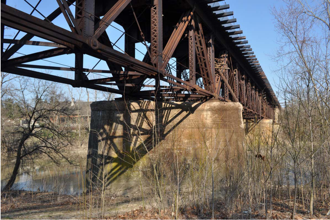
The PRR Bradford Line bridge across the Scioto River looking east. This bridge abutment was heavily damaged during the Great Flood of 1913. It was repaired and 107 years later still stands.
